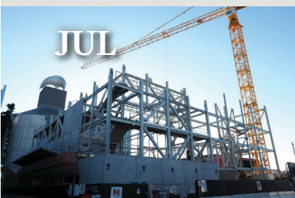
70% of structural steel completed, stage concrete bases poured, 50% of precast panels erected and assembly of the theatre roof began.
