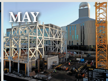
Passed the sixth month mark of the construction period, since dismantling the Moana Fisheries building in 2014.
