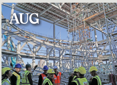
Theatre roof lifted onto the building in three sections. Structural steel and precast panels completed. By the end of August, Level 3 was at 90% completion, Level 4 at 50% completion and the ground floor was at 85% completion.
