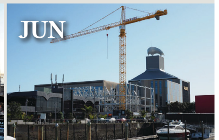
First two sections of steel erected to the fly tower, foundations for the structure were completed and the first of the precast panels were erected.
